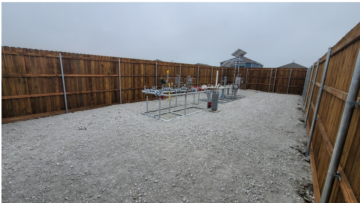
Figure 2: Regulation & Odorization Components
