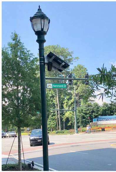
Solar & Existing Pole
