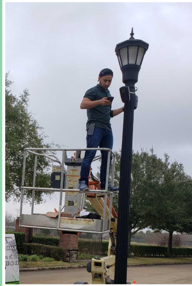
Electric & Existing Pole
